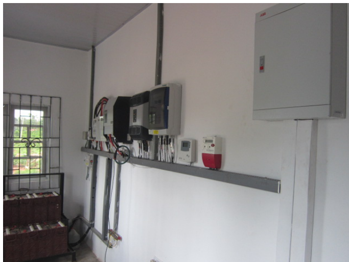
Fig 8 PV Generator Room
