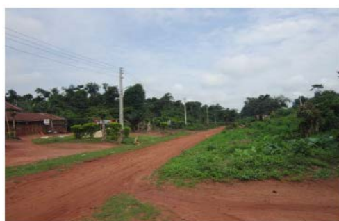
Emuhun LV Distribution poles
